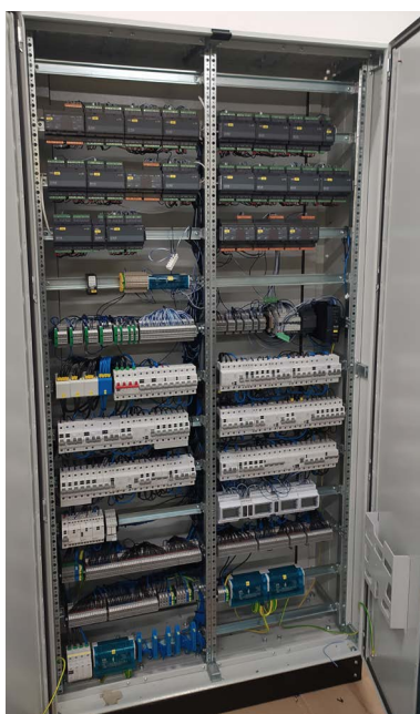
Finished distribution board
